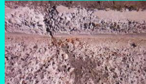
Figure 5.12 Cracking and spalling of concrete
