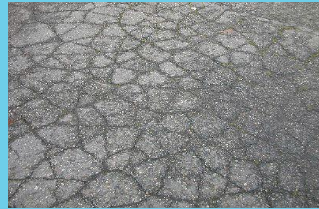
Figure 3.33 Asphalt Alligator Cracking
