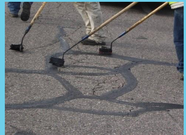
Figure 5.12 The climate creates challenges for maintaining infrastructure such as the need to seal cracks in pavement
