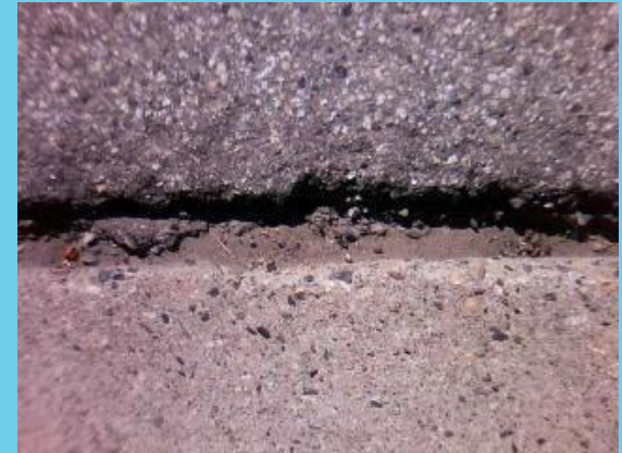
Figure 3.35 Pavement and Gutter Separation
