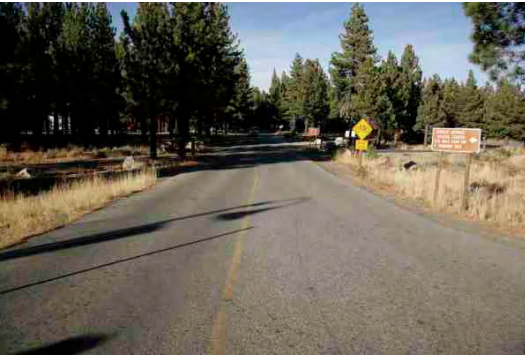
Photo #2 Notes Condition photo
