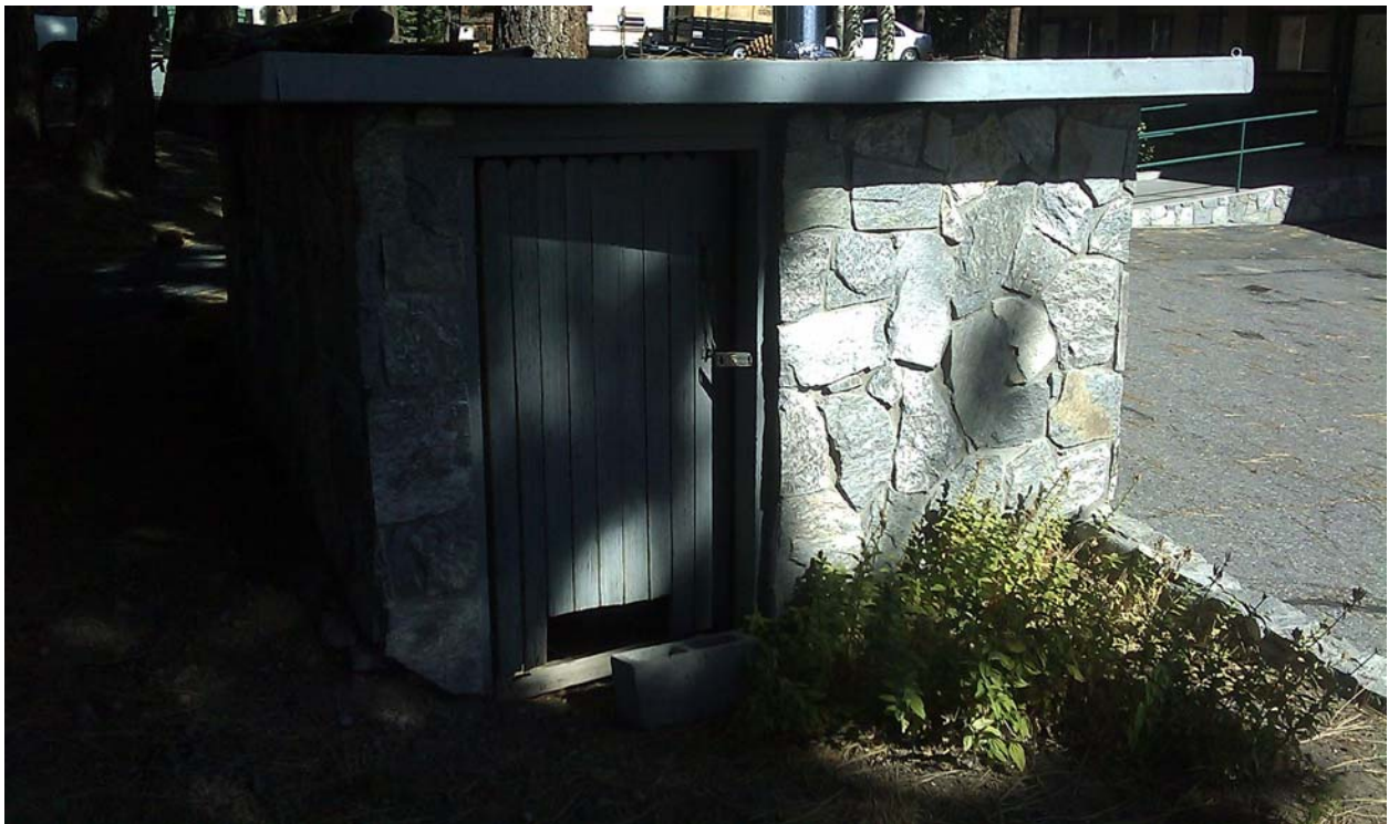
Photo 24. View of entry to abandoned pump house adjacent to former outdoor Jacuzzi located between the east and west buildings of Royal Pines Resort.
