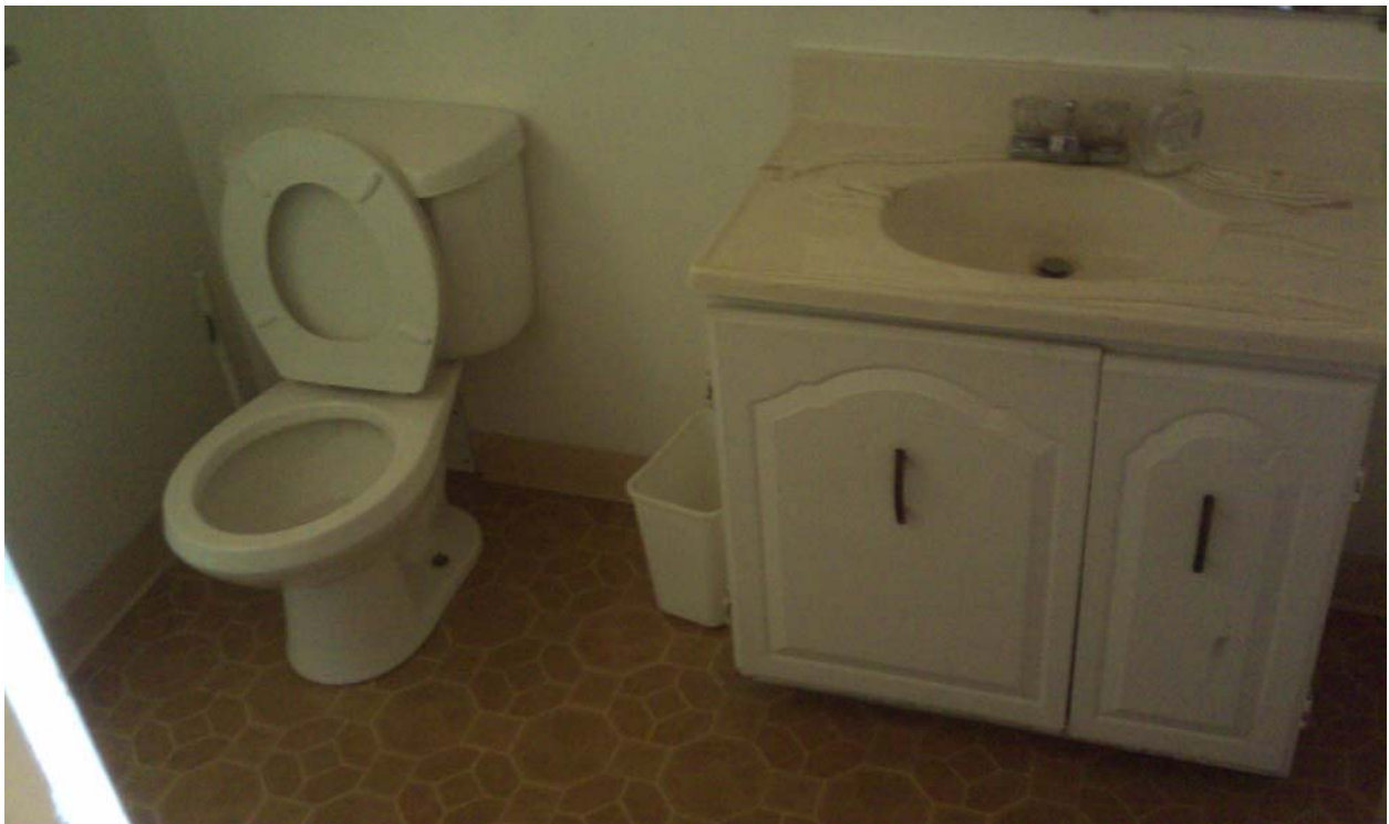
Photo 12. View of bathroom floor inside Unit 11 composed of PACM.
