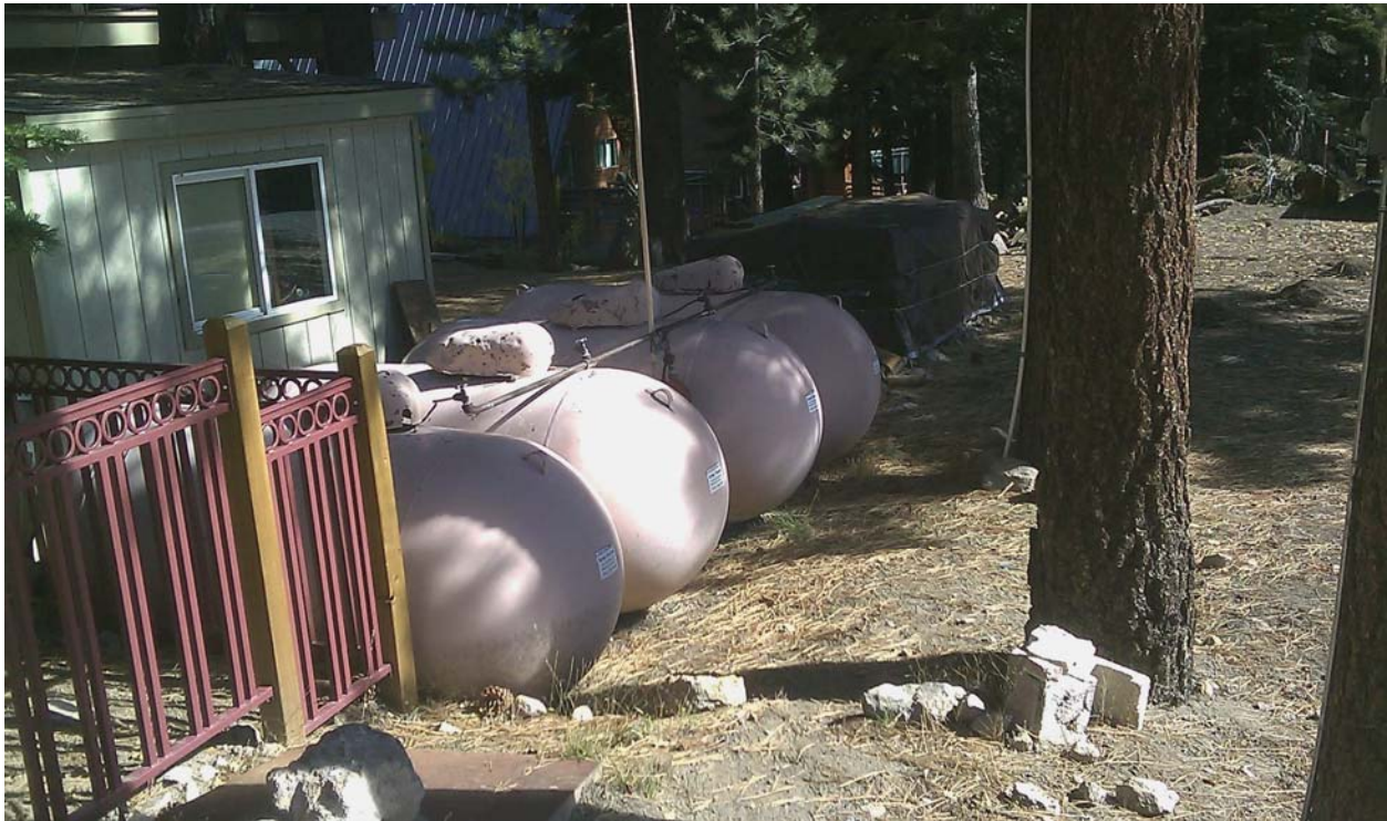
Photo 63. View looking northeast at four "offsite" propane tanks located on northern property line.
