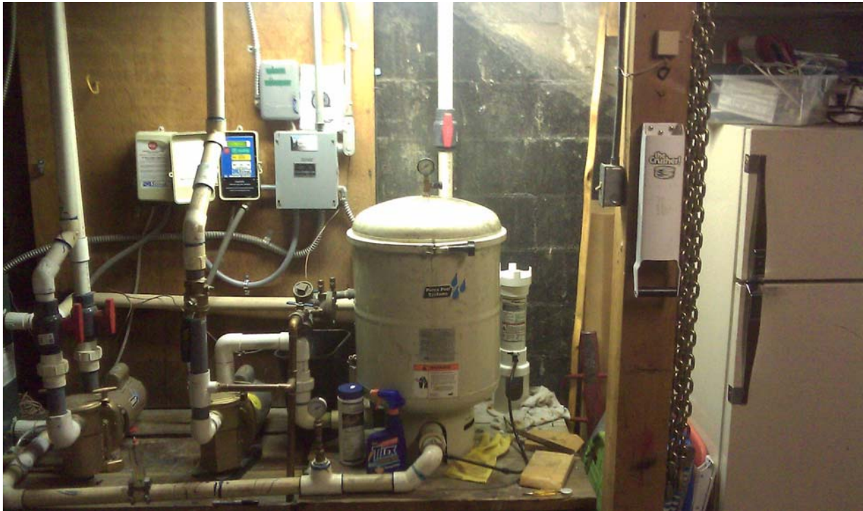
Photo 31. View inside Swiss Chalet maintenance room at Jacuzzi pump system on east wall.
