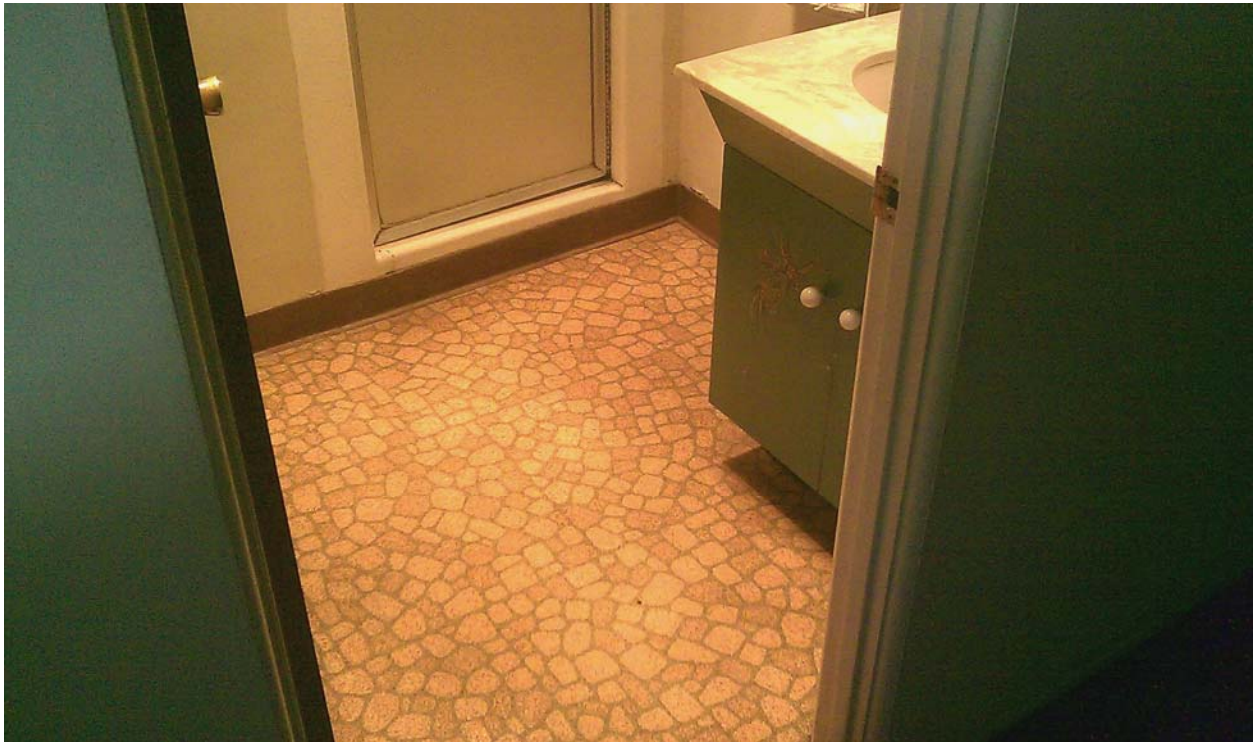
Photo 45. View of floor tiling inside Unit 22 composed of PACM.
