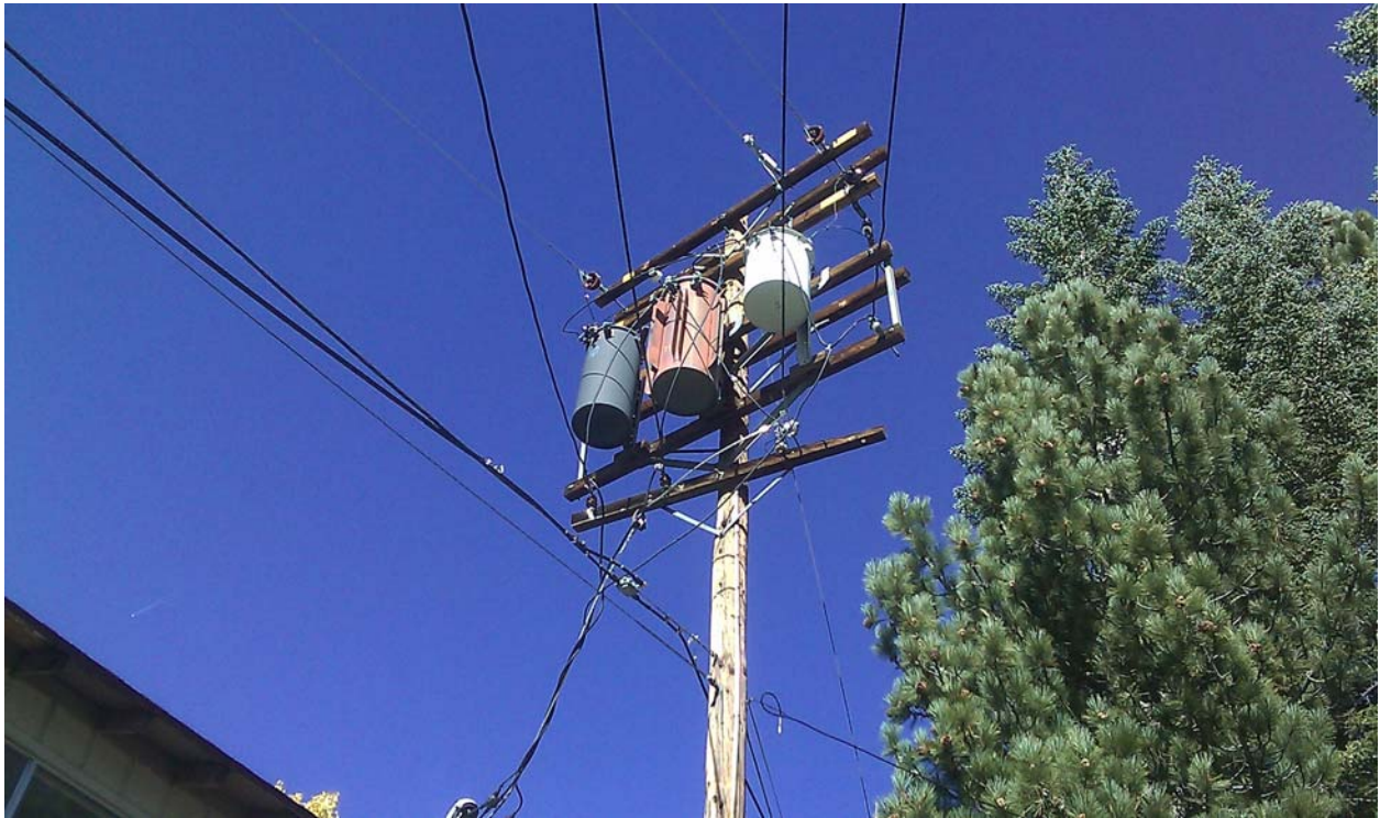
Photo 51. View of 3-phase electrical transformers mounted on SCE power pole 1592948E, all of which are likely to contain polychlorinated biphenyls (PCBs).
