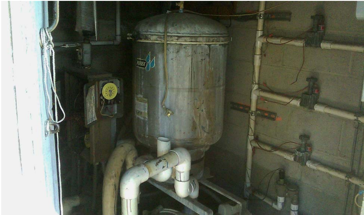
Photo 25. View inside Jacuzzi pump house.
