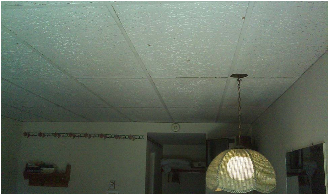
Photo 41. View of ceiling board inside Unit 6 composed of PACM.
