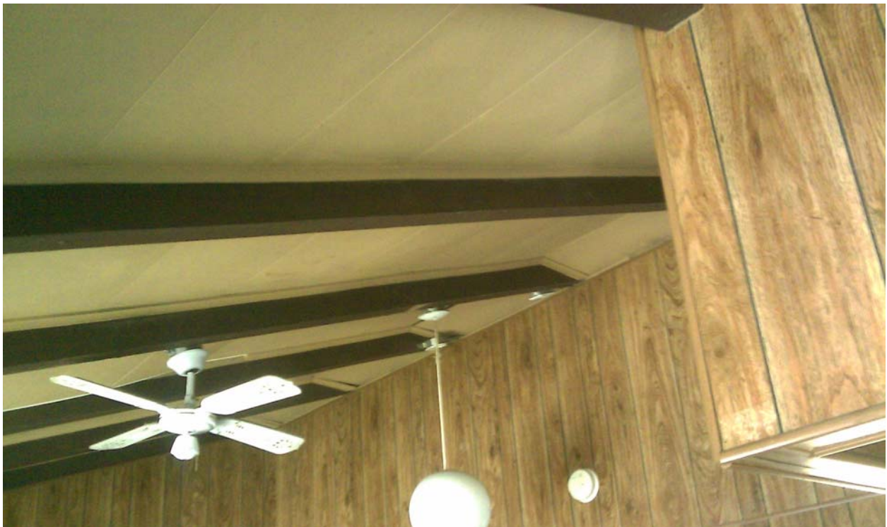
Photo 10. View of ceiling inside Unit 11 composed of potential asbestos-containing material (PACM).
