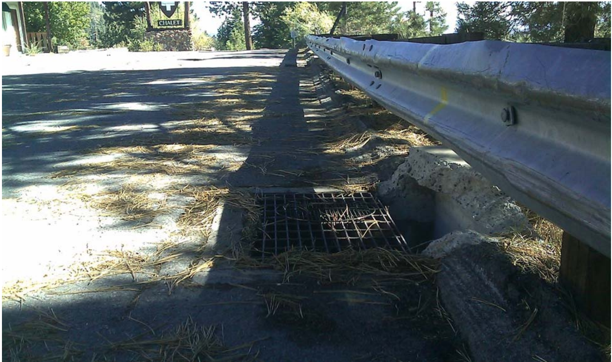
Photo 55. View looking close-up at western stormdrain inlet located on View Point Road south of Swiss Chalet.
