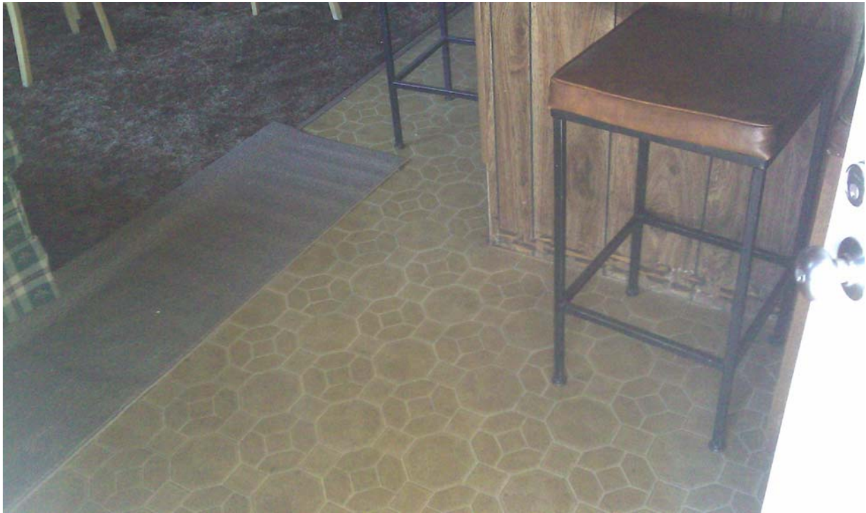
Photo 11. View of kitchen floor inside Unit 11 composed of PACM.
