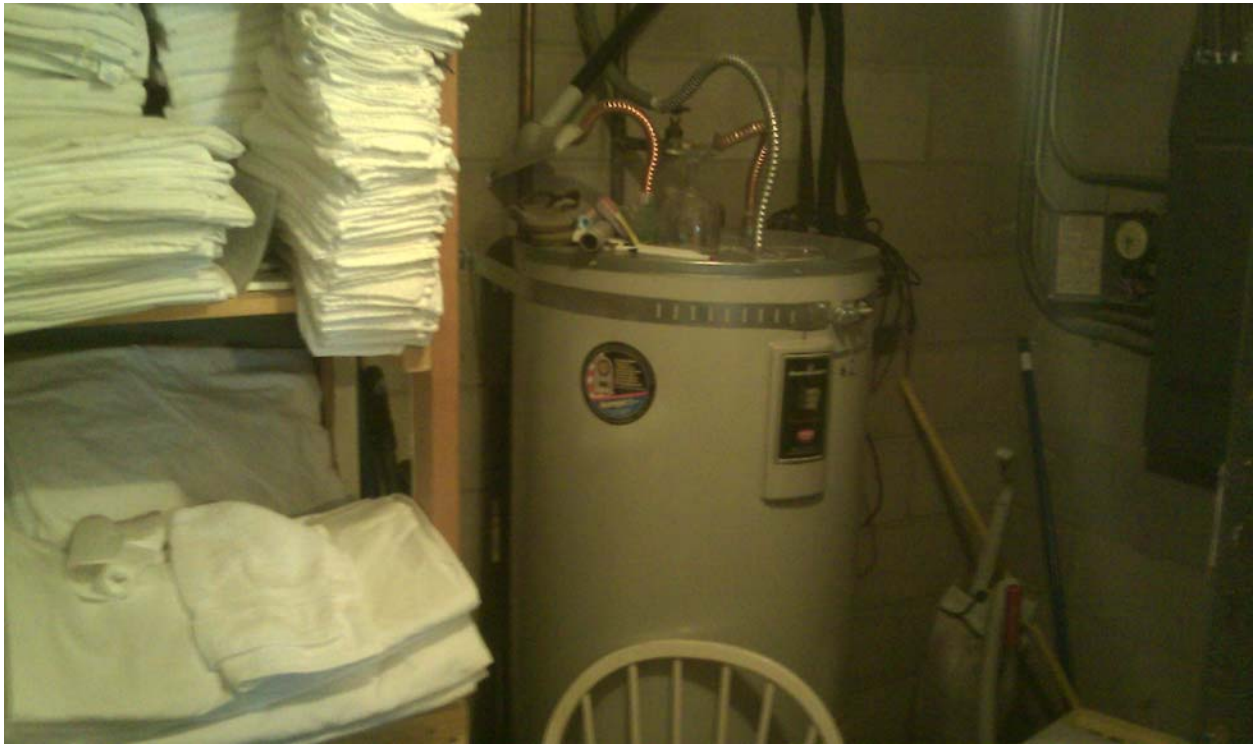
Photo 39. View of hot water heater inside laundry room.
