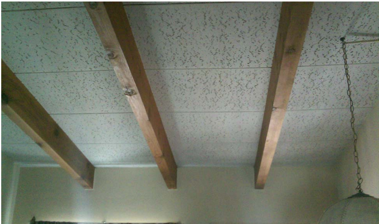
Photo 44. View of ceiling board inside Unit 22 composed of PACM.
