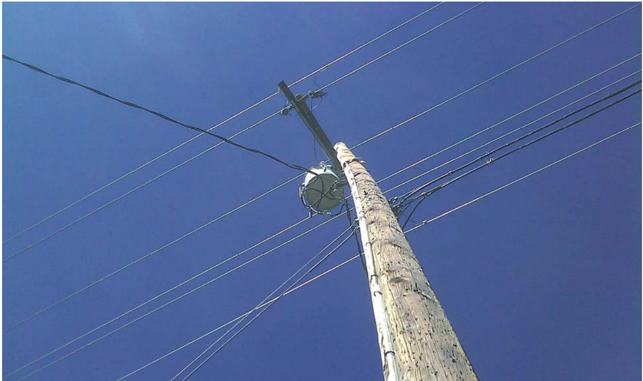
Photo 53. View of single-phase electrical transformer mounted on SCE power pole 2179738E, which is unlikely to contain PCBs.
