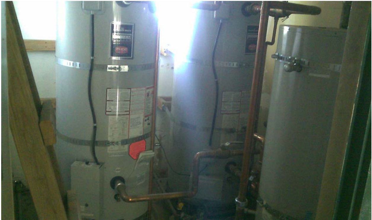
Photo 19. View of hot water heaters inside east building maintenance room.
