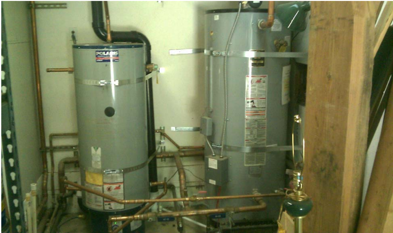
Photo 7. Close-up view looking west at hot water heaters inside maintenance room.
