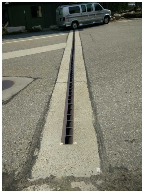
If drains for melting snow are plugged, runoff from rain-on-snow events may not drain properly and can lead to flooding.
